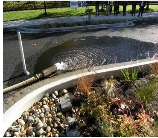
A fire hose demonstrates the pervious asphalt and rain garden in action.
