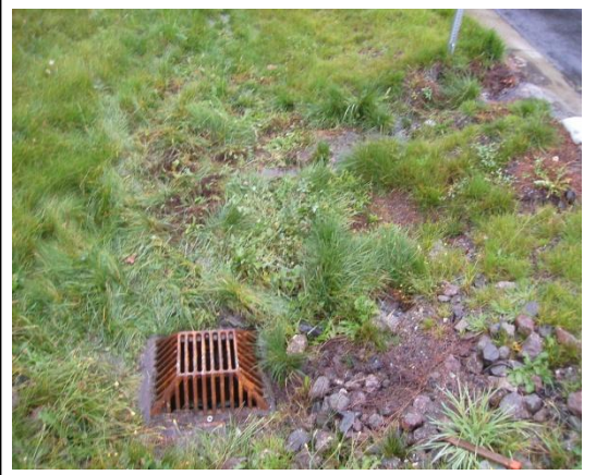
Before post-construction adjustments
