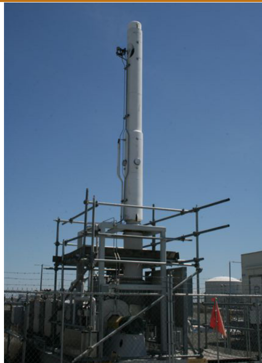
An extension will add 23 ft., to an exhaust stack similar to this one at 296-P-49, which is planned for use at C-107.
