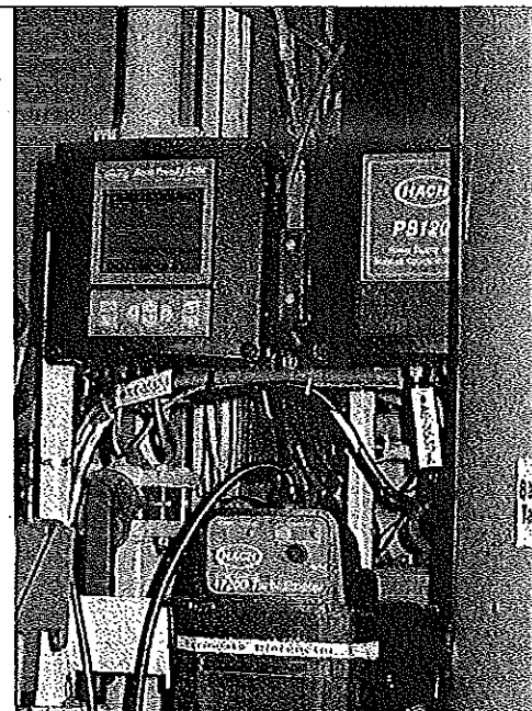
PHOTO #:08 DATE: SEPTEMBER 18, 2009 TAKEN BY: MARK HENDERSON FILE No.: IMG_013 DESCRIPTION: AWTS – TURBIDIMETER
