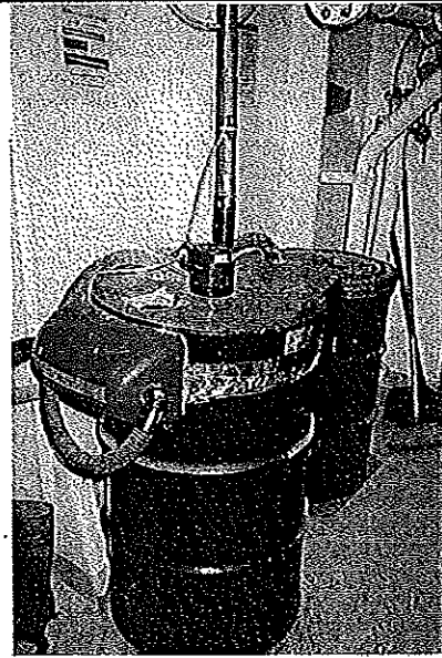
PHOTO #:18 DATE: JULY 19, 2009 TAKEN BY: AMY JANKOWIAK FILE No.: P8080018 DESCRIPTION: FLUORESCENT BULB CRUSHER (BOTTOM) - MERCURY REMOVAL SYSTEM
