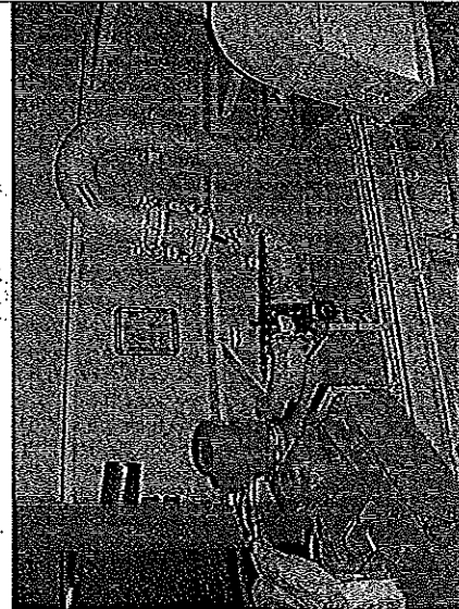
PHOTO #:24 DATE: JULY 19, 2009 TAKEN BY: AMY JANKOWIAK FILE No.: P71900 DESCRIPTION: BLACK/GRAY WATER DISCHARGE PORT (PADLOCKED)
