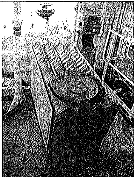
PHOTO #:11 DATE: JULY 26, 2009 TAKEN BY: MARK HENDERSON FILE No.: IMG_1123 DESCRIPTION: OWS FACET SPARE FILTER
