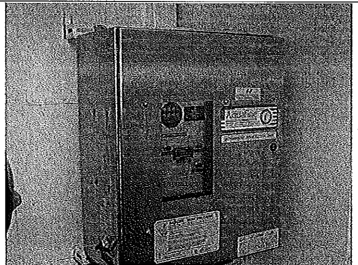
PHOTO #:08 DATE: JULY 26, 2009 TAKEN BY: MARK HENDERSON FILE No.: IMG_1115 DESCRIPTION: UV DISINFECTION SYSTEM CONTROL BOX
