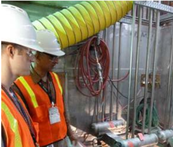
Ecology's Robbie Biyani and Dieter Bohrmann observe construction of the leak detection system in the pre-treatment facility at the Hanford tank waste treatment plant.
