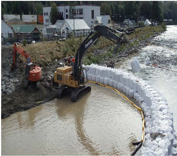
Crews remove the coffer dam after finishing cleanup work at the Skykomish cleanup site.
