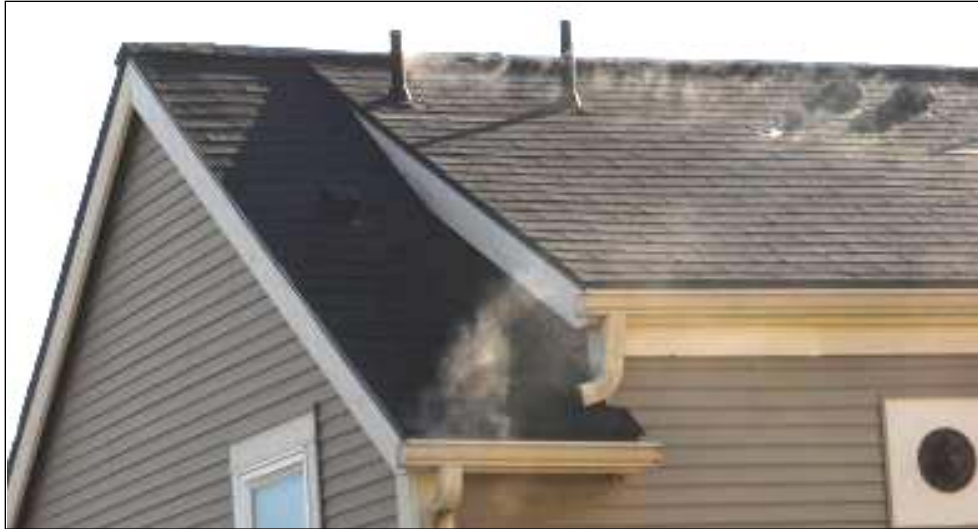
Smoke testing of the stormwater system in the New Holly development in Seattle identifies a home with an illicit connection.
