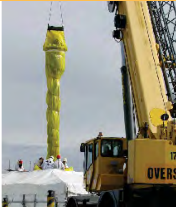
A broken pump is removed from double-shell tank AN-106, which will receive waste from SST C-107. A new pump will be inserted and used to support waste retrieval.
