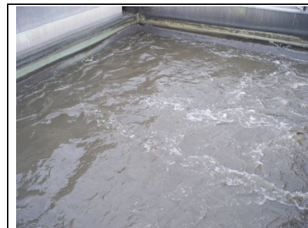
Dunes Facility's Headworks after installation of IP's new treatment system.
