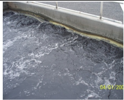
Black water at the city of Moses Lake's Dunes Facility's Headworks
