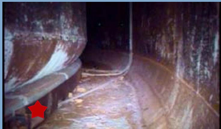
Inside the annulus, or space between the primary and secondary tanks, of tank AY-102, the steel stabilizing ring at the base of the inner tank is 6 1/2 inches tall, 3/8 inches thick, and supports the base of the inner tank.
