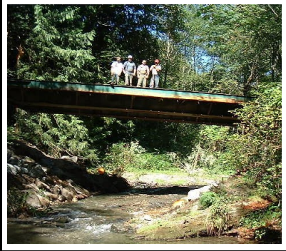
Top: Culvert that was replaced Bottom: Skagit Fisheries staff stand on the new bridge
