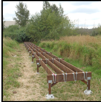
After months of working in mud, the ground dries and a boardwalk begins to take shape.
