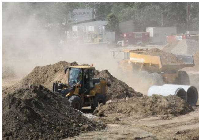
Visible dust on a construction site is against state law. Arsenic and lead in dust can pose a health risk.
