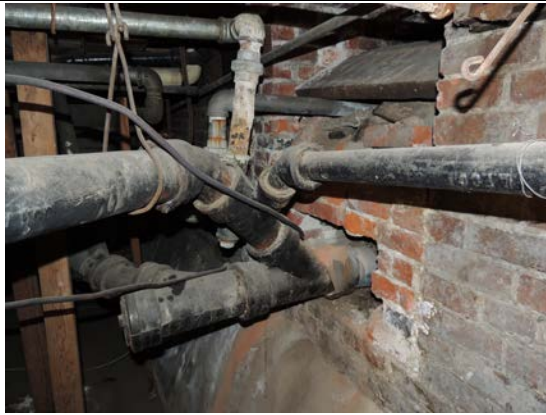
Web of pipes under the historic building where the illicit connection was found Photo credit: Pullman Stormwater Services
