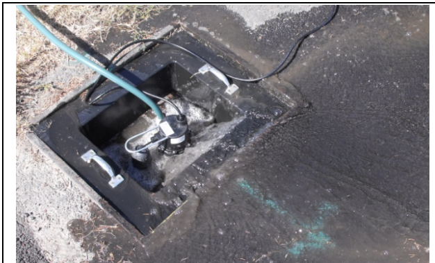
Soapy water flowing into a catch basin where the pump transfers it to the sanitary sewer
