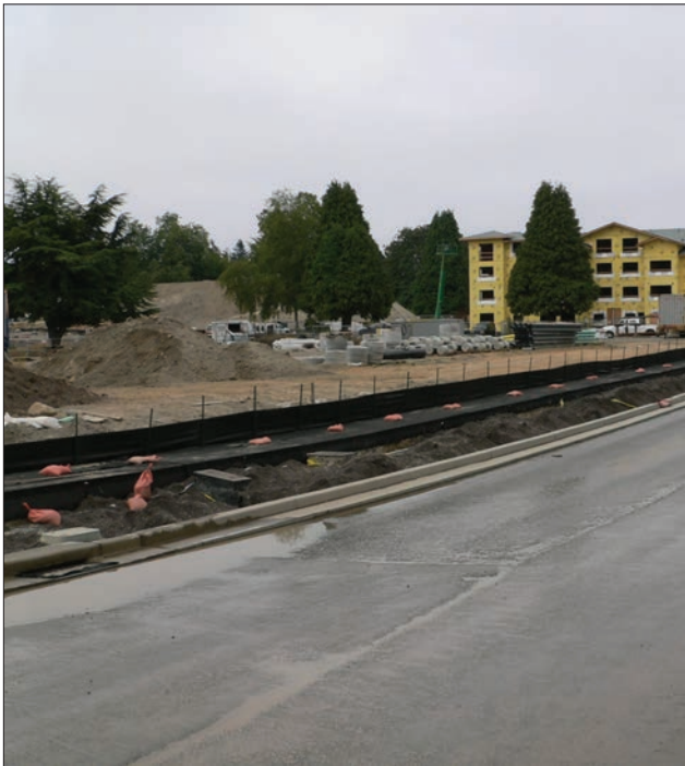
FIGURE 4.6.9 Filter fabric placed under this pervious concrete sidewalk is wrapped over the pavement and secured to protect the installation during construction. Source: Curtis Hinman
