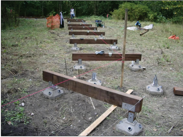
FIGURE 4.8.3 - FOOTBRIDGE WITH MINIMAL EXCAVATION FOUNDATION Construction of a foot-bridge utilizing minimal excavation foundations at the Auburn Environmental Park in Auburn, Washington. Source: AHBL, Inc.
