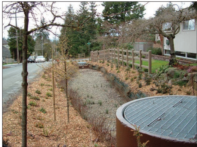
FIGURE 4.4.10 Catch basin inlet. Source: Photo by Curtis Hinman
