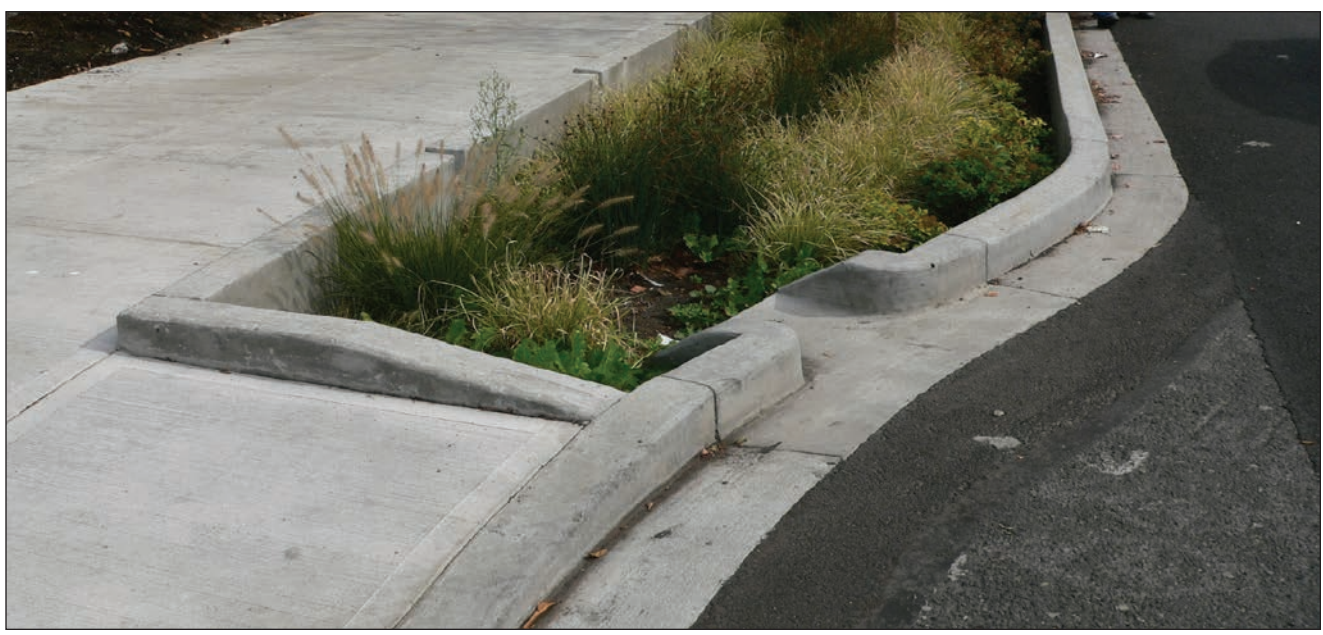
FIGURE 4.4.8 Typical curb cut details Source: Photo by Curtis Hinman Illustration courtesy of the Bureau of Environmental Services, City of Portland, OR.
