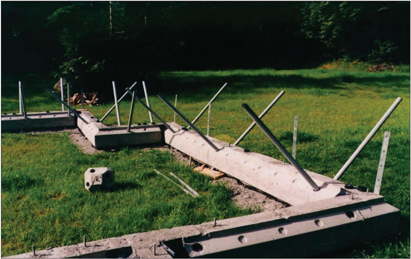
FIGURE 4.8.6 - WALL TYPE MINIMAL EXCAVATION FOUNDATION Pier type foundation. Source: Pin Foundations, Inc.
