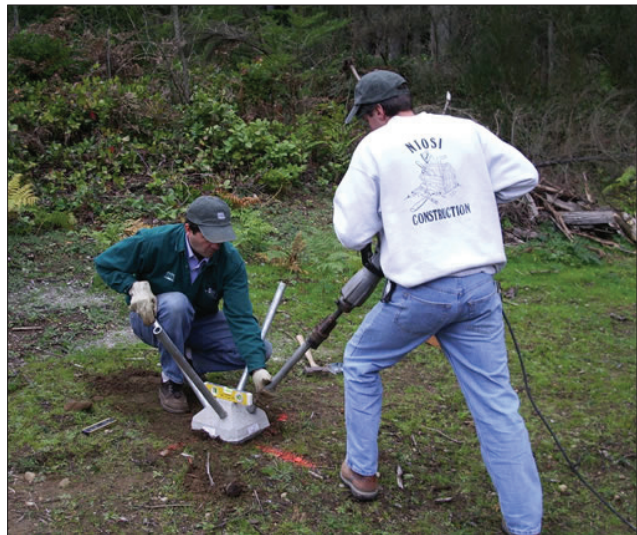
FIGURE 4.8.8 - PILE DRIVING Driving of pile with automatic hammer Source: Pin Foundations, Inc.
