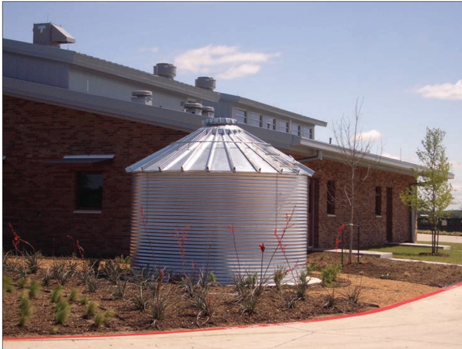
FIGURE 4.9.3 - CISTERN USED TO MEET NON-POTABLE WATER NEEDS Rain water harvest system used to meet the non-potable water demands of the Denton Fire Station. Source: Innovative Water Systems, LLC
