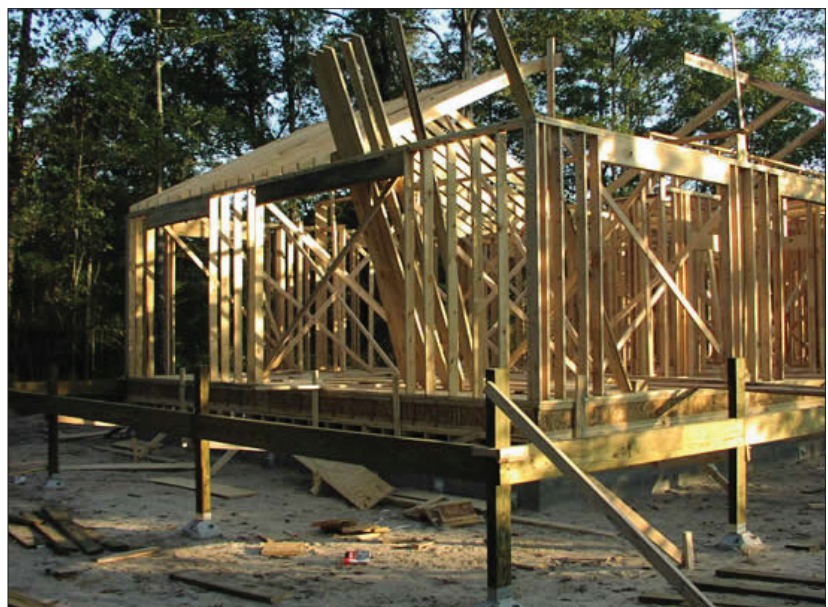
FIGURE 4.8.7 - FLAT SITE CONSTRUCTION ON PIERS Construction of a single-family home on piers on a relatively flat site Source: Pin Foundations, Inc.
