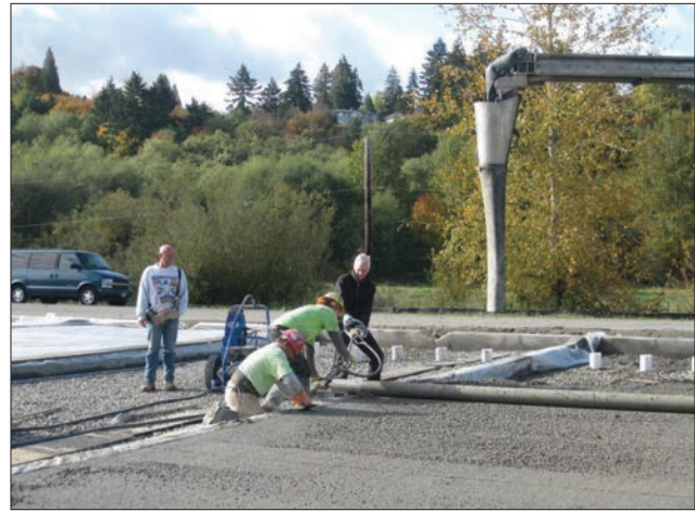
FIGURE 4.6.10 Hydraulically operated Bunyan screed compacts and provides the finished elevation in one preparation. Source: SvR Design, courtesy of Low Impact Development Technical Guidance Manual for Puget Sound (2012)
