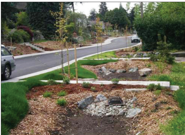
FIGURE 4.4.13 Bioretention outlet structure photo and drawing providing elevation drop. Source: AHBL, Inc. courtesy of Low Impact Development Technical Guidance Manual for Puget Sound (2012) Photo by Curtis Hinman
