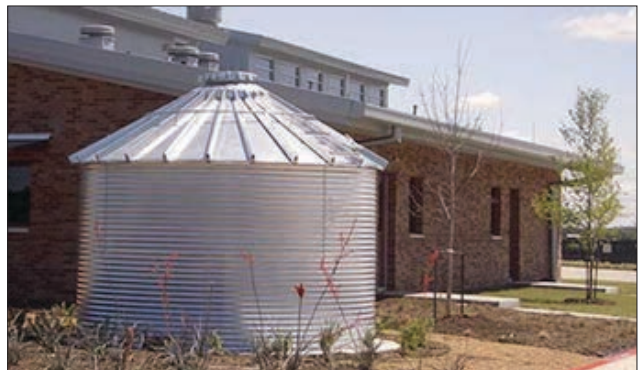
FIGURE 3.13 RAIN WATER COLLECTION SYSTEM Rain water collection system on a fire station in the dry climate of Denton, Texas. Source: Innovative Water Solutions, Austin, TX
