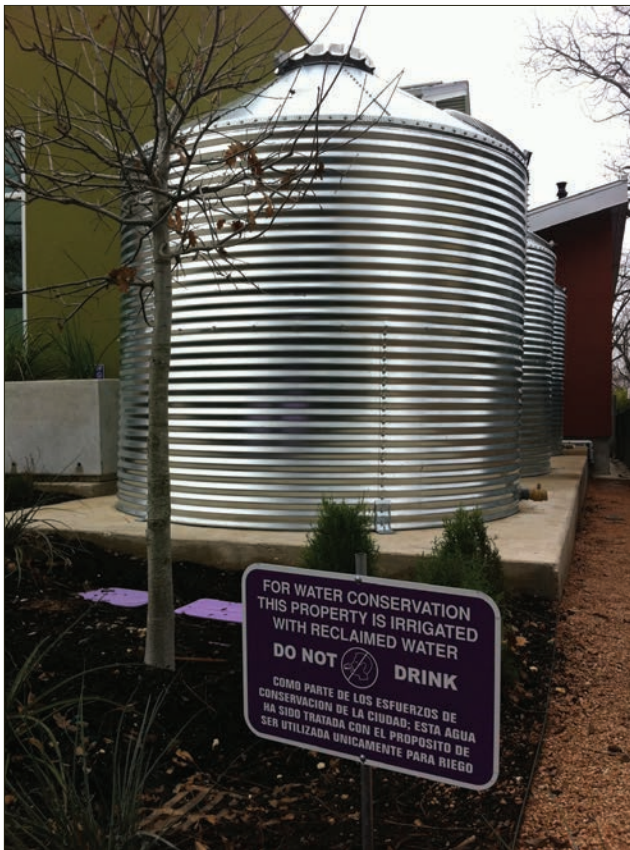
FIGURE 4.9.2 - CISTERN USED TO MEET IRRIGATION NEEDS Rain water harvest system used to meet the irrigation demands at the Eagle Veterinary Hospital in San Antonio, Texas. Source: Innovative Water Systems, LLC
