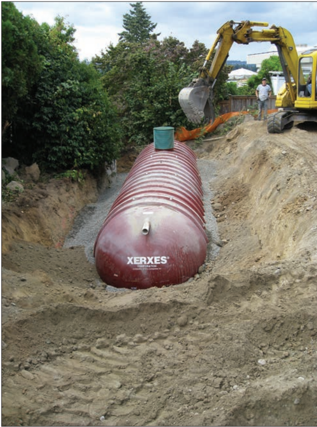
FIGURE 4.9.4 - EXCAVATION FOR AN UNDERGROUND CISTERN Excavation associated with the installation of an underground rain water harvest system supporting the non-potable water demands of a residential structure. Source: David Hilgers, R Miller, Inc.
