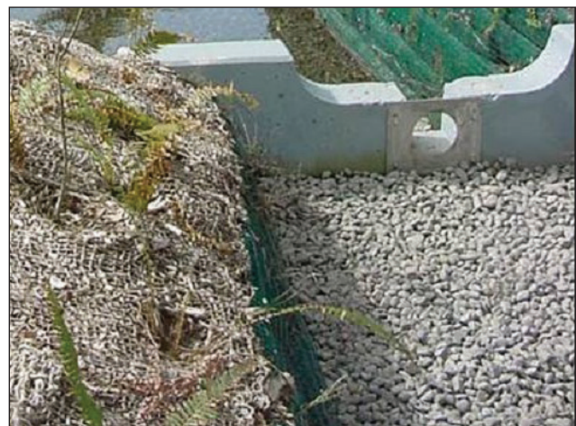
FIGURE 4.4.19 Aggregate mulch is used in the high gradient bioretention swale. Plants are installed through the aggregate mulch and into the BSM below. Source: Photo by Curtis Hinman
