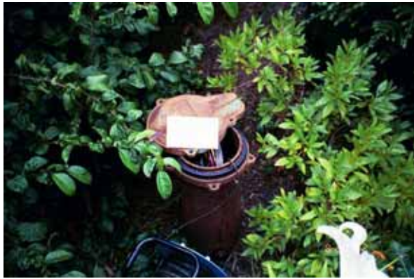
Figure 2-4. Typical water level measurement point. Note the electronic well probe is visible just below the wellhead.
