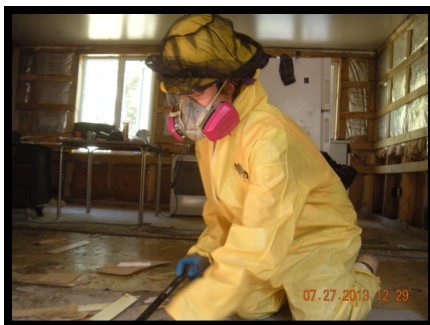
Gutting and taking out flooring and sopping wet insulation in a Galena home.
