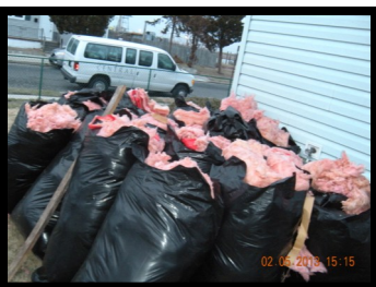
Bags of wet insulation pulled from a crawlspace.
