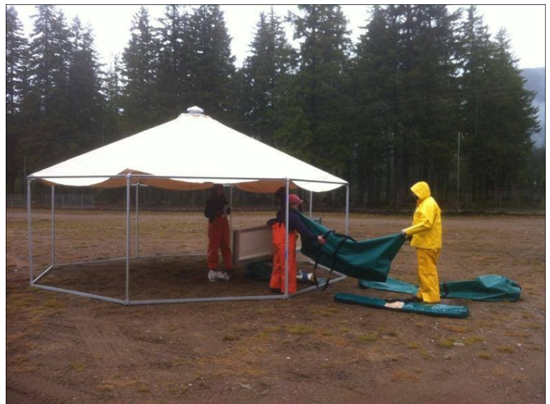
The Port Angeles crew constructs a Yurt in Darrington at the responder tent camp. Photo courtesy of Luke Wigle.
