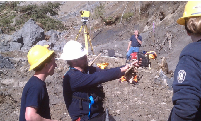
Dallas Barron, Ernie Farmer, and Morgan Gilchrist assist with LiDAR installation. The yellow device in the background is part of the LiDAR equipment used to monitor shifts in the hillside above rescuers.
