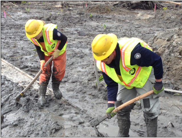
WCC crew members assist excavators and SAR crews by digging trenches at the debris field.
