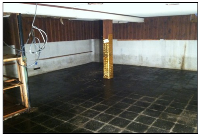
Damaged home after completed work
