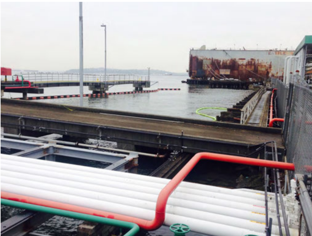
Photo 2. BP Terminal seawall parallel to loading rack on right, green boom to capture any sheen or floating product on West Waterway is a safety measure. Foreground is piping for on-loading and off-loading petroleum from barges or ships at West Waterway. Left is barge and ship dock with Elliott Bay is in background.
