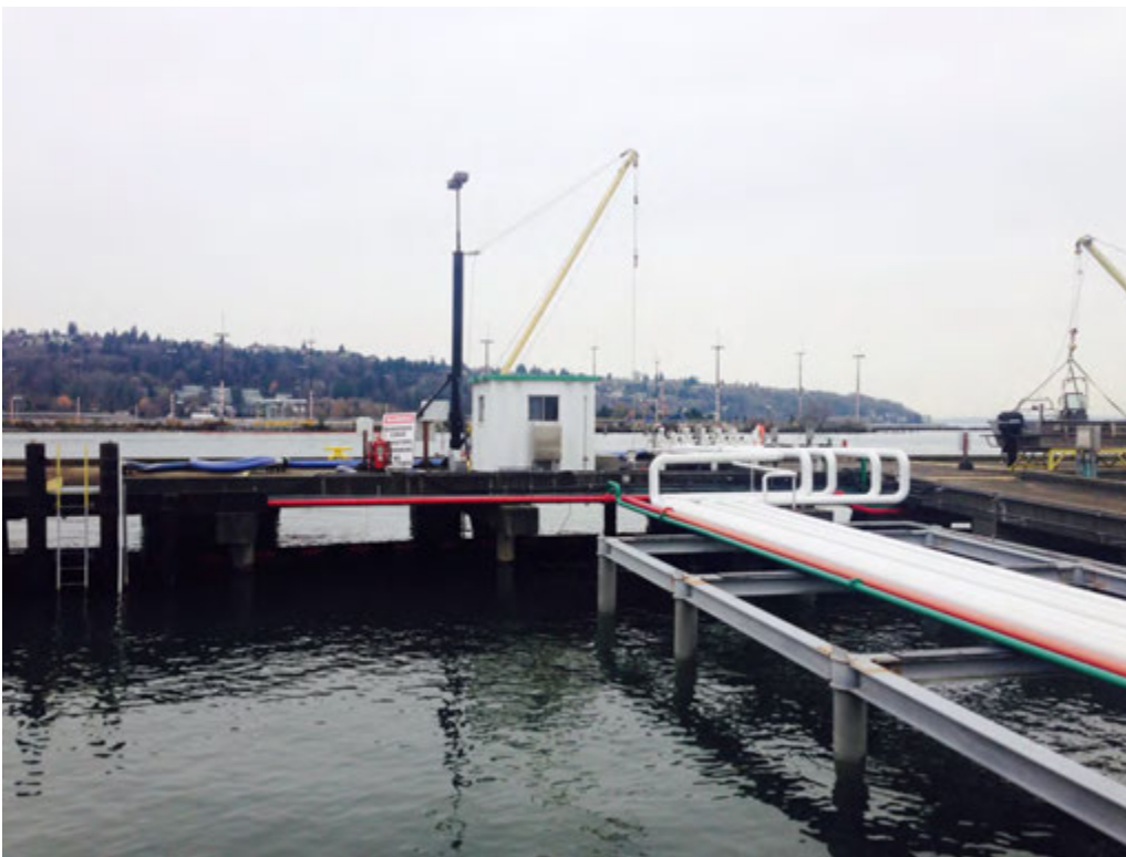
Photo 4. BP Terminal continuation of photo 2 showing on-loading and off-loading petroleum fuels piping and dock at West Waterway looking westward in distance is the north edge of West Seattle.
