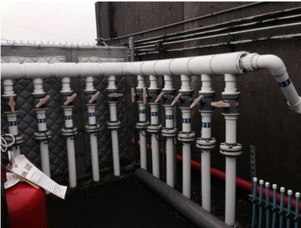
Photo 8. BP Terminal detail for the Soil Vapor Extraction Remediation System showing 11 individual well control valves and piping. Blue airlines to right were installed as a contingency in case additional remedial technologies, such as air sparging, would be needed to meet site cleanup objectives. This system is removing petroleum vapors from soil and groundwater for subsurface cleanup action.
