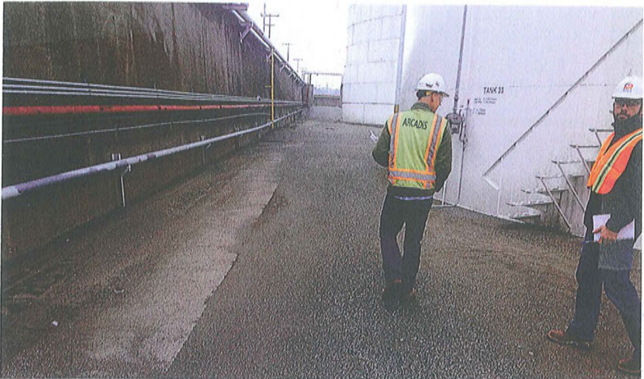
Photo 3. KMLT Above ground petroleum Storage Tank No. 33 at B Yard with containment wall and piping on left with two Arcadis consultants conducting the site inspection.
