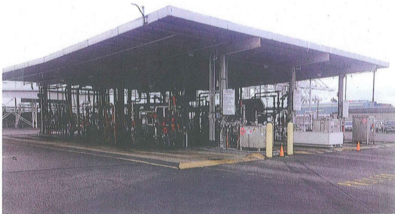
Photo 1. KMLT illustrating a petroleum fuels loading rack.
