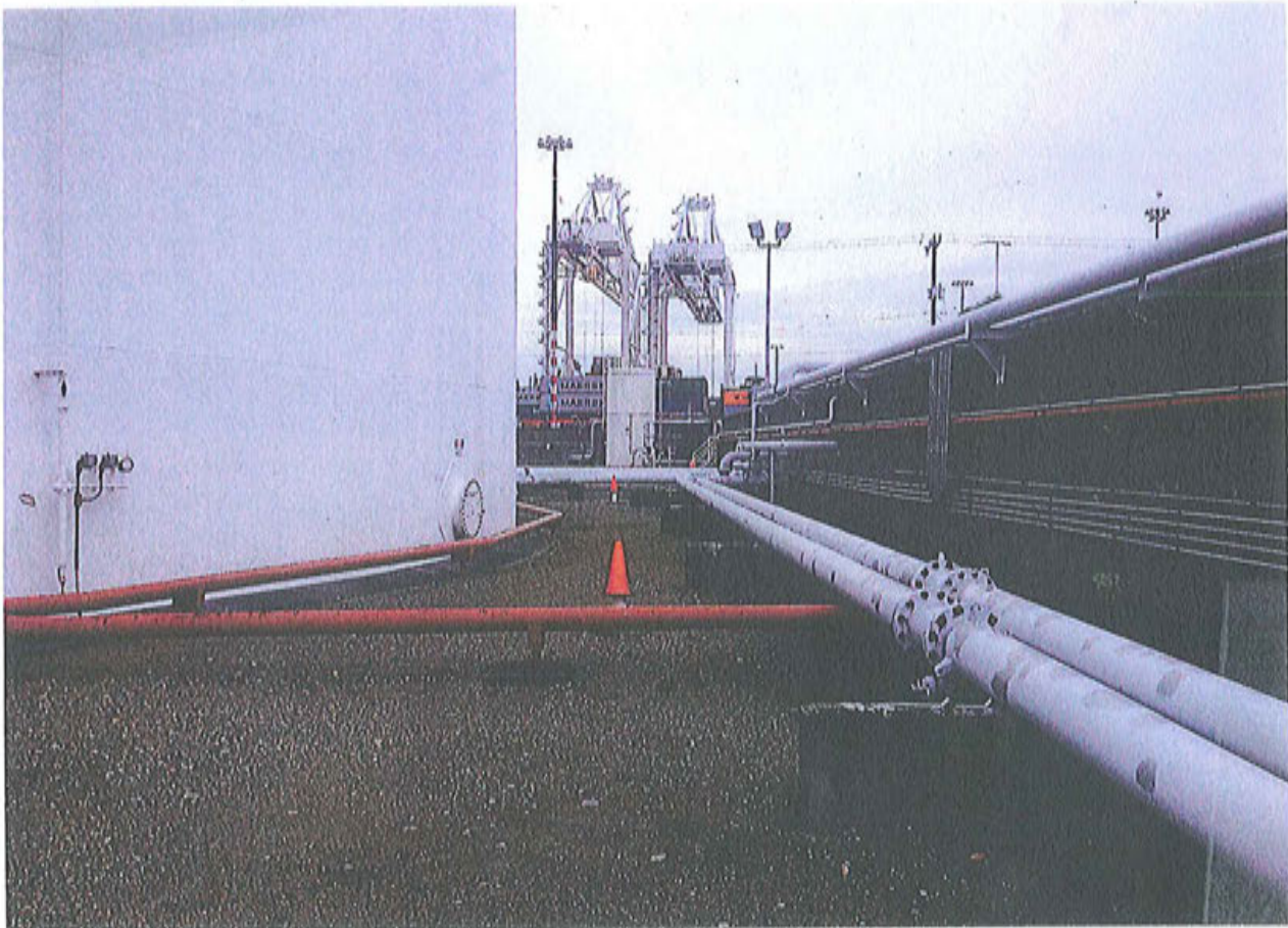
Photo 6. KMLT Above ground petroleum Storage Tank and supply piping with containment wall to right.
