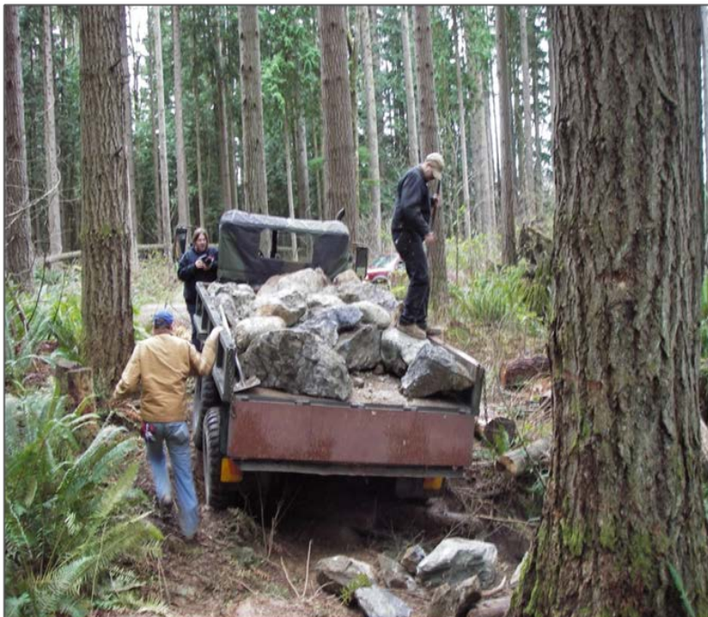
Volunteers provided thousands of hours of labor and the machinery necessary for trail construction.
