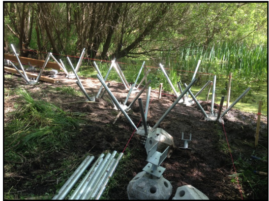
Above: These footings are known as "diamond pier footings" and will hold the boardwalk in place.
