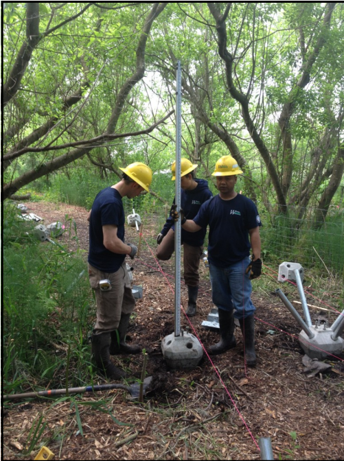
Left: Members work with a transit to find the correct elevation for the footing. Four metal pipes are inserted into each footing.
