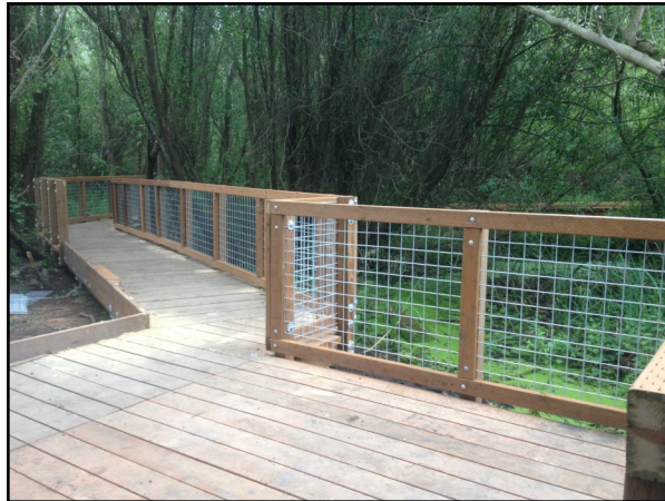
Finished railings along boardwalk ensure the environment is protected from people wanting to wander through the native plants
