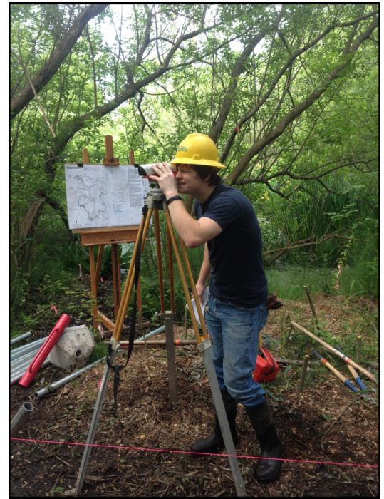
Surveying the land where the boardwalk is being constructed. Precise measurements are taken to ensure a level boardwalk.
