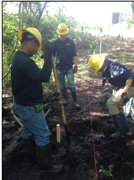
Crew members preparing to place low impact concrete footings along surveyed lines. These will become the support system of the boardwalk.
