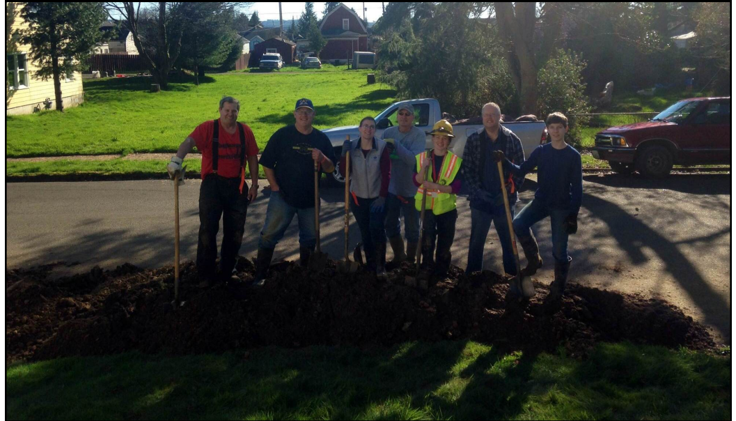
Hardworking volunteers and team leader Ashley Matelski with mud removed from backyard. Photos courtesy of Ashley Matelski.
