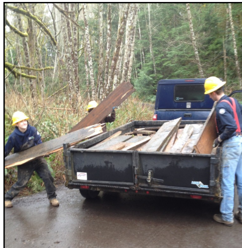
2. Rip up old boardwalk. Scrape and level old trail. Remove 6-8 inches of mud from most of it.
