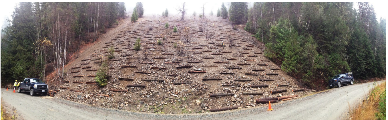
Old school slope restoration in Metaline Falls by the Walla Walla Spike and the Spokane Spike AmeriCorps Crews. This is the start of a 42 year watershed restoration project that Seattle City Light must complete to recertify their Dam on the Pend Oreille River. (Photos submitted by Adam Hein's and Greg Dunbar's crews).
