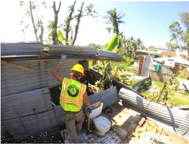
WCC AmeriCorps member Ashtyn Moss helps demo an unsalvageable structure at a weekend service event. Photo submitted by Adeline Wisernig.
