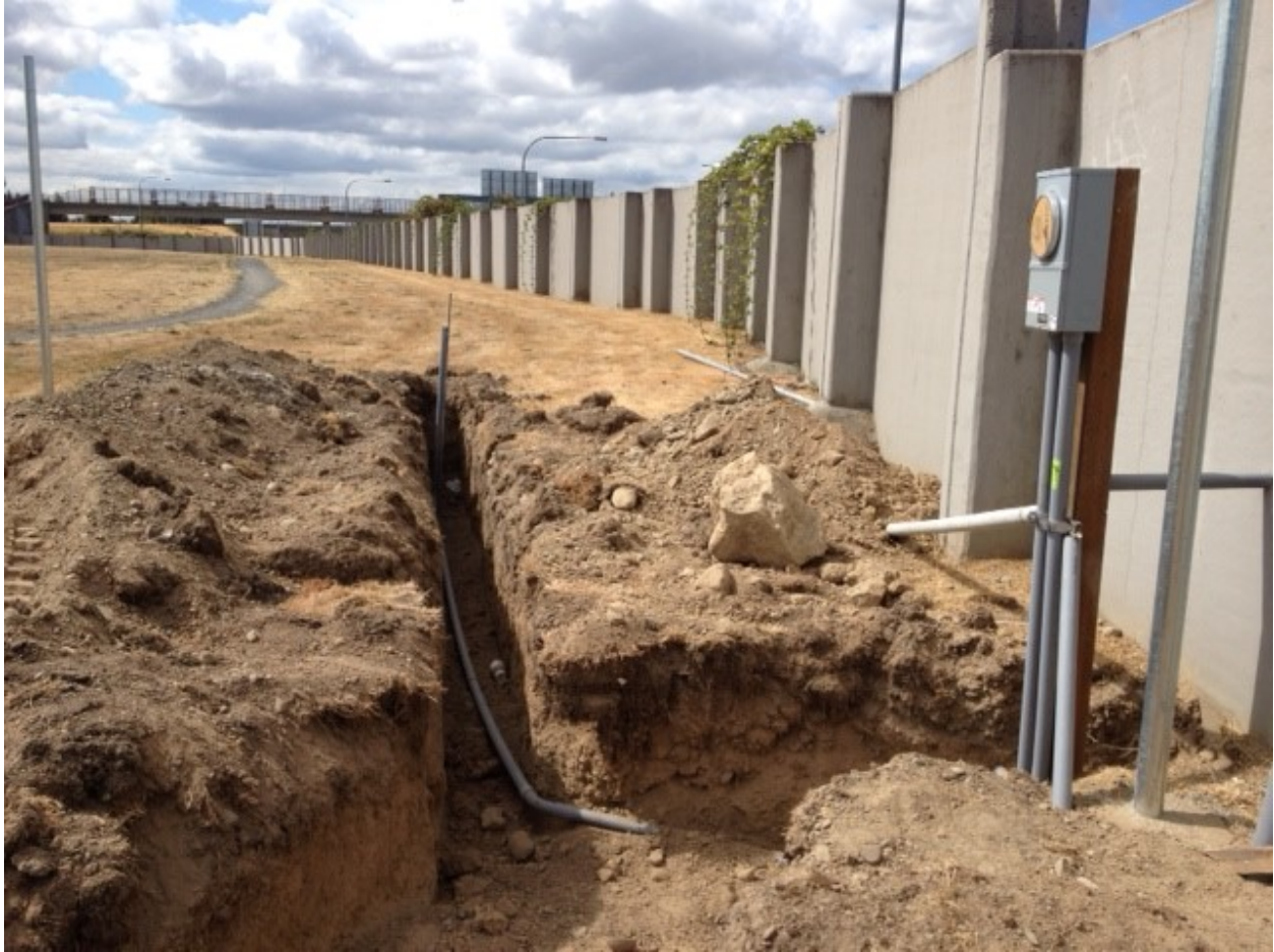
Figure 2: Electrical installation at the Tacoma-S. 36th St. Near-road location
