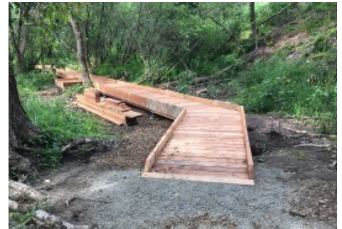
The completed boardwalk at Yesler Swamp. Photo by Friends of Yesler Swamp.
