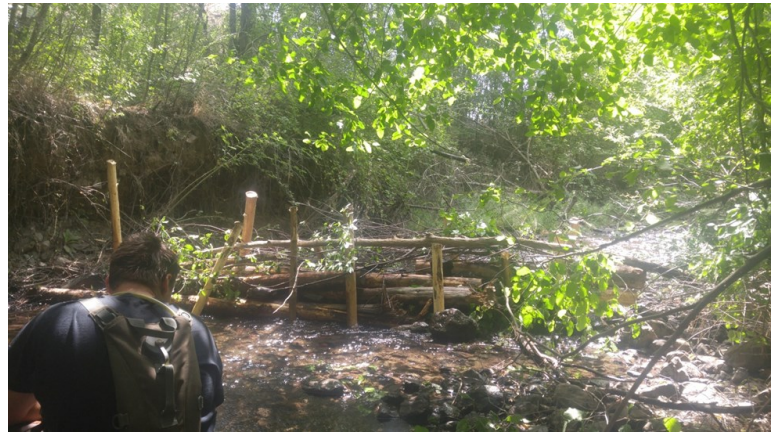
Sam Richardson admiring the ALS-Mid Channel structure. Photo submitted by Hayden Lucia.
