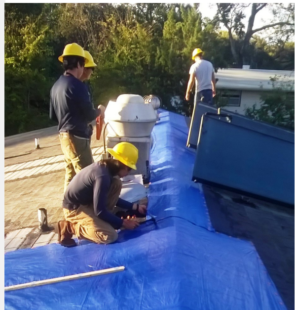
WCC members perform tarping on a residential roof. Photo submitted by WCC.
