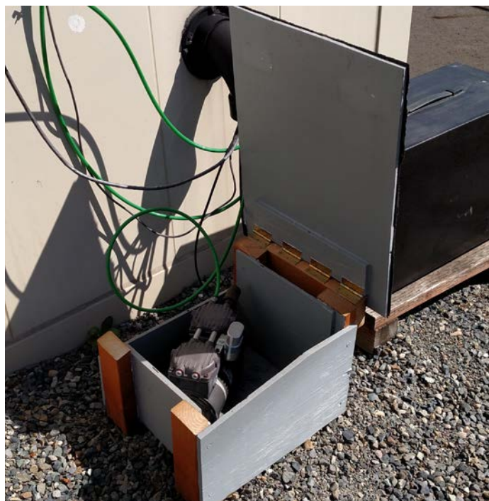
Figure 3: Photo of outdoor pump enclosure (photo courtesy of PSCAA)
