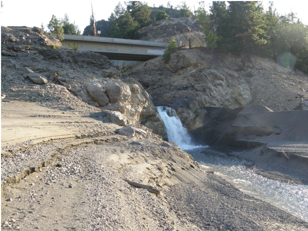
Figure 3-19. Rimrock Reservoir drawdown resulting in a passage barrier at the South Fork Tieton River below Forest Service Road 1200 (Photo by William Meyer, WDFW).
