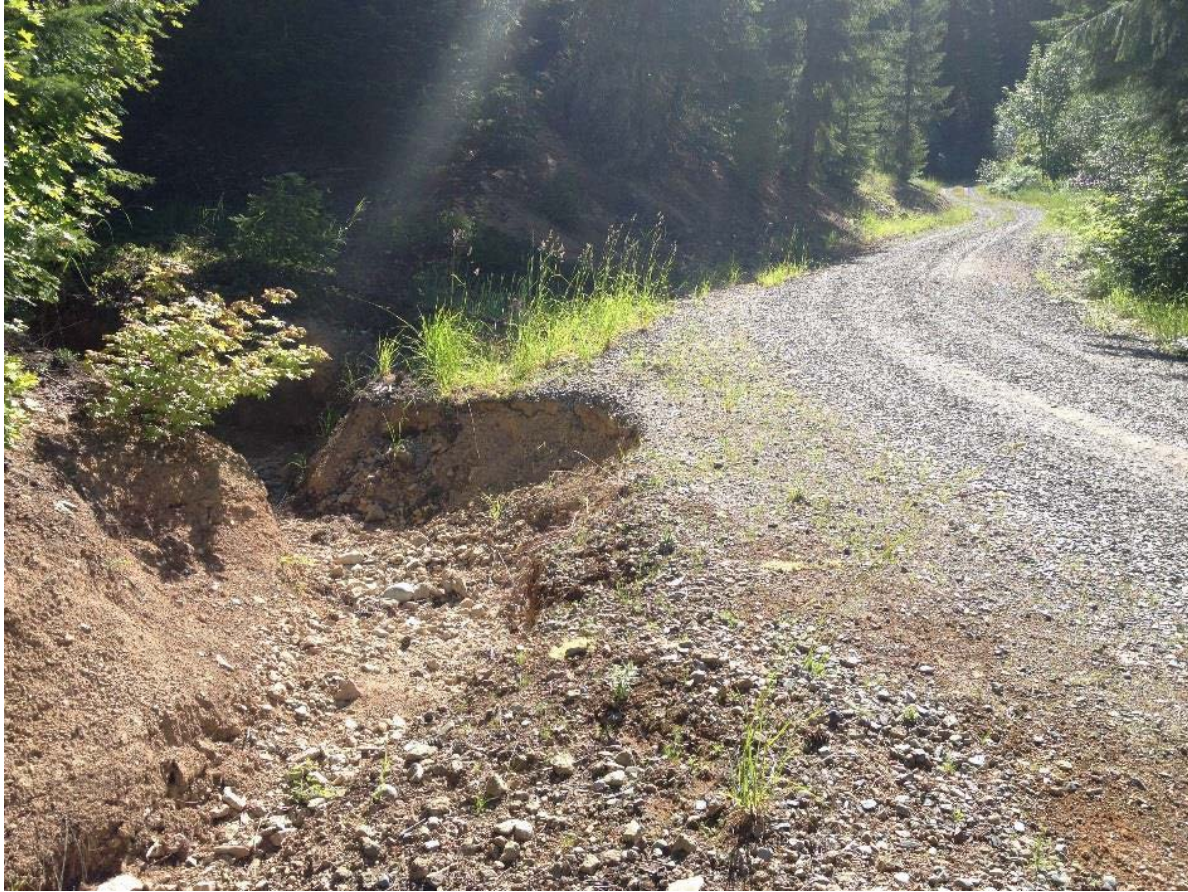
Figure 3-17. Erosion along lower section of Forest Service Road 4600.
