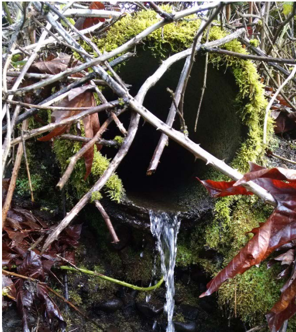
Figure 22. Stormwater event effluent from outlet to hillside and Salmon Creek.
