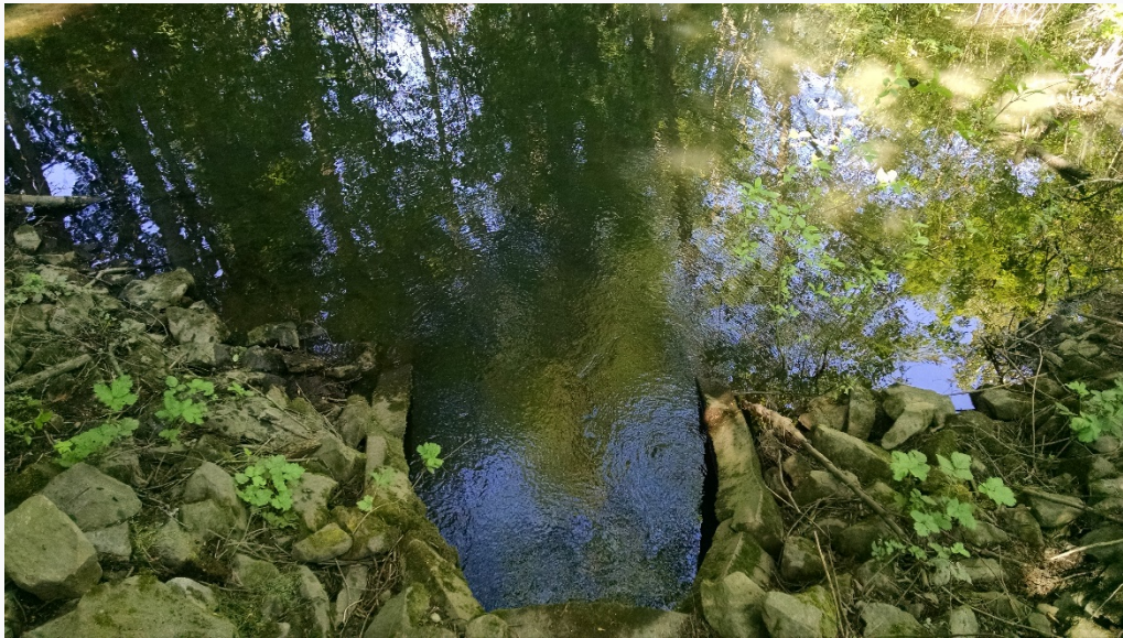
Figure 24. Looking downstream from above at the CC_CAPT site at detention basin culvert inlet.
