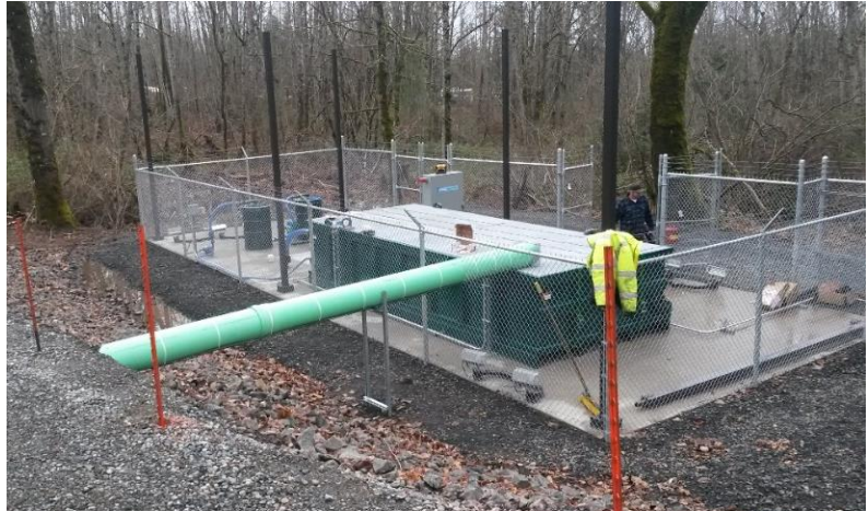
Figure 1. Treatment system installed to reduce pH and remove arsenic from the seepage.
