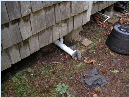
Figure 1. An example of an OSS failure. A pipe sends household wastewater directly into the ground without treatment.
