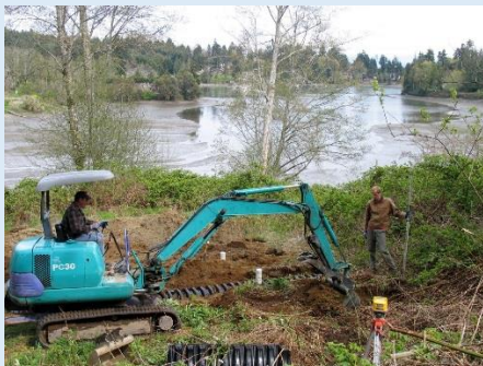
Figure 2. An excavator works on onsite sewage system replacement project along the Puget Sound.
