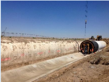
Figure 1 Building infrastructure like this siphon brings 164,000 ac-ft of surface water for irrigation to replace water from a declining aquifer in the Odessa sub-area, one of the most productive agricultural regions in the country.
