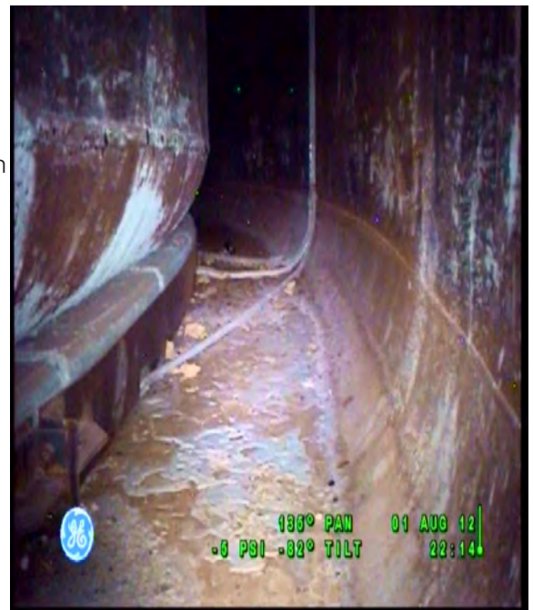
Waste on floor of outer shell in AY-102 annulus
