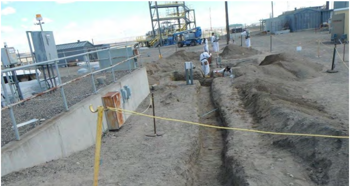
2015 photo showing several workers digging trenches at AY-102 in preparation for waste retrieval. Many of the trenches throughout the tank farms must be hand dug, to avoid hitting unmapped pipes or conduit.
