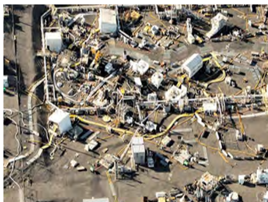
Surface infrastructure that was in place while workers were retrieving waste from the C-Farm tanks.
