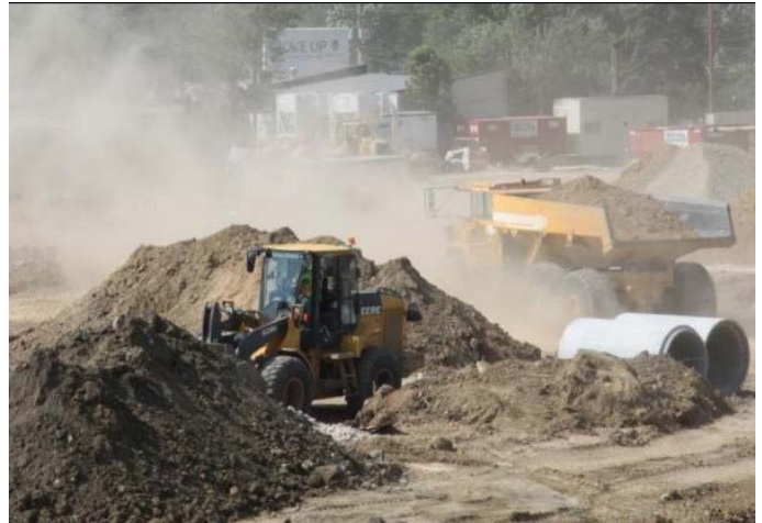
Visible dust on a construction site is against state law. Arsenic and lead in dust can pose a health risk.
