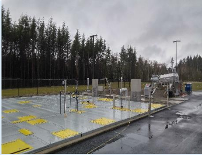
Figure 1 Membrane bioreactor treatment facilities significantly reduce nutrients in wastewater and produce a much cleaner effluent safe for discharge. Photo Credit: Port Gamble S'Klallam Tribe.
