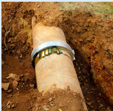
Figure 3: Sewer pipe taking waste to a POTW. Photo credit: Bidgee.
