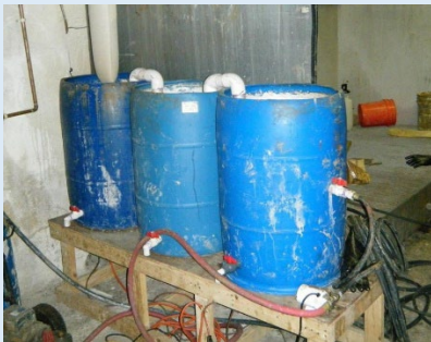
Figure 2: Facility improperly treating wastewater in 55-gallon containers. This treatment isn't legal.
