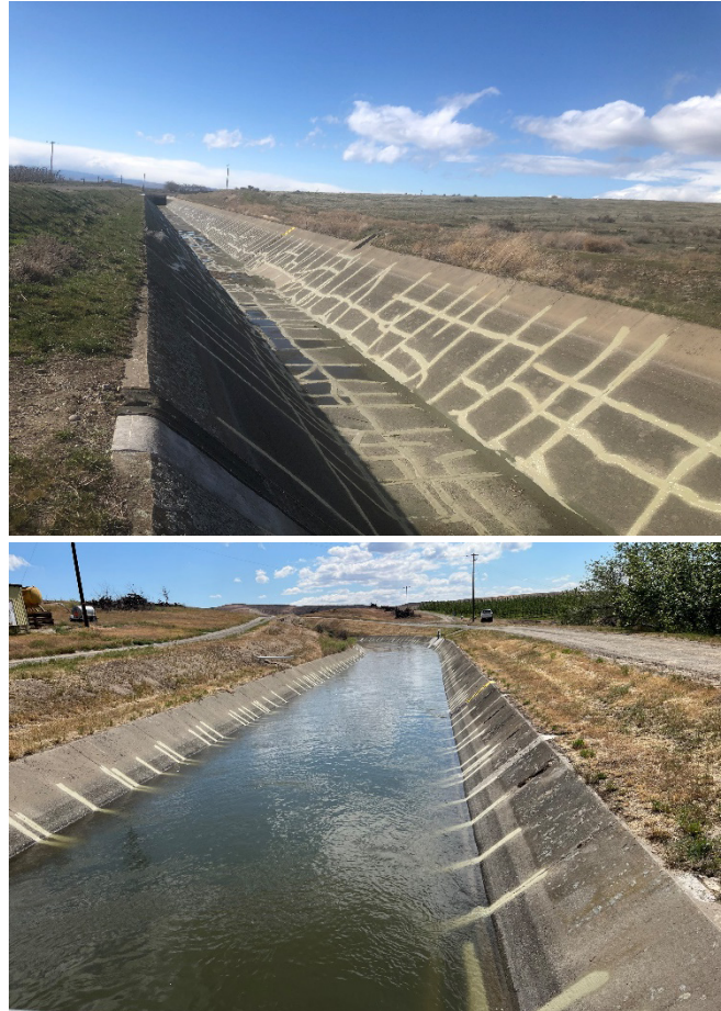
Roza main canal sealing complete. Dry (top) and full (bottom) canal comparison.
