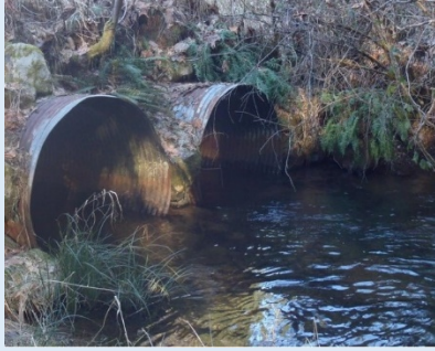
These barrier culverts on Bush Creek near Elma have been replaced, opening 8.2 miles of forested habitat for fish.
