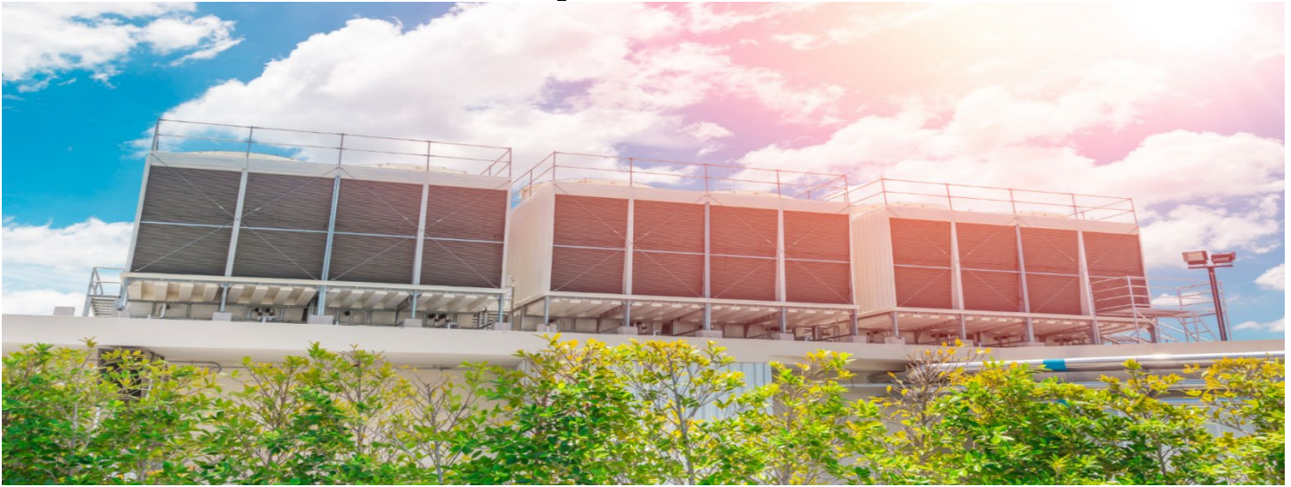
Figure 1. Large air-conditioning unit containing hydrofluorocarbons (HFCs)
