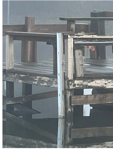
Example 2. Pier-mounted staff gauge
