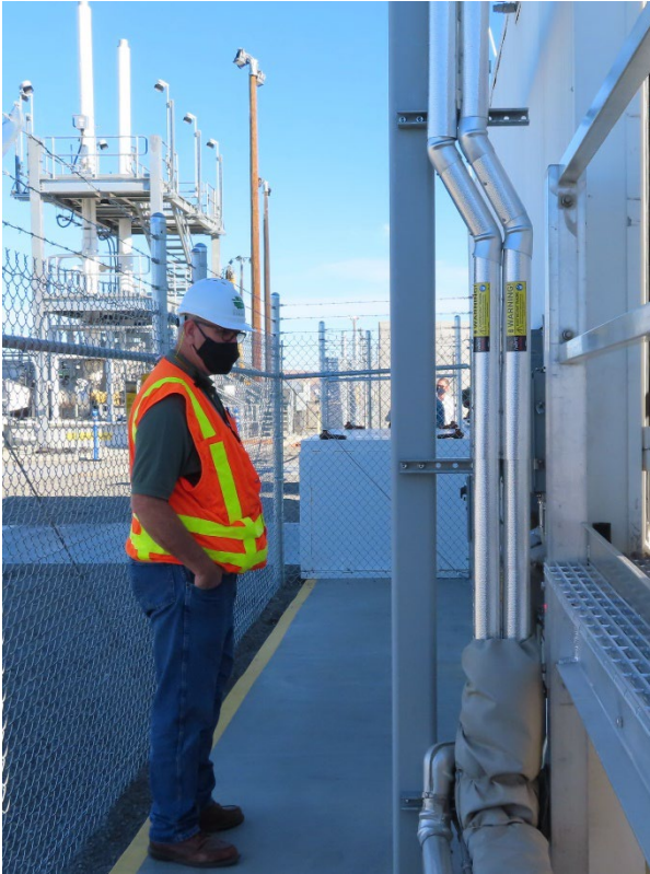
Jay Decker (the Science and Engineering Unit Supervisor for the Nuclear Waste Program) inspects part of the Tank-Side Cesium Removal System (TSCR) at Hanford. Ecology regularly inspects dozens of Hanford site facilities. TSCR began pretreating tank waste in January 2022.
