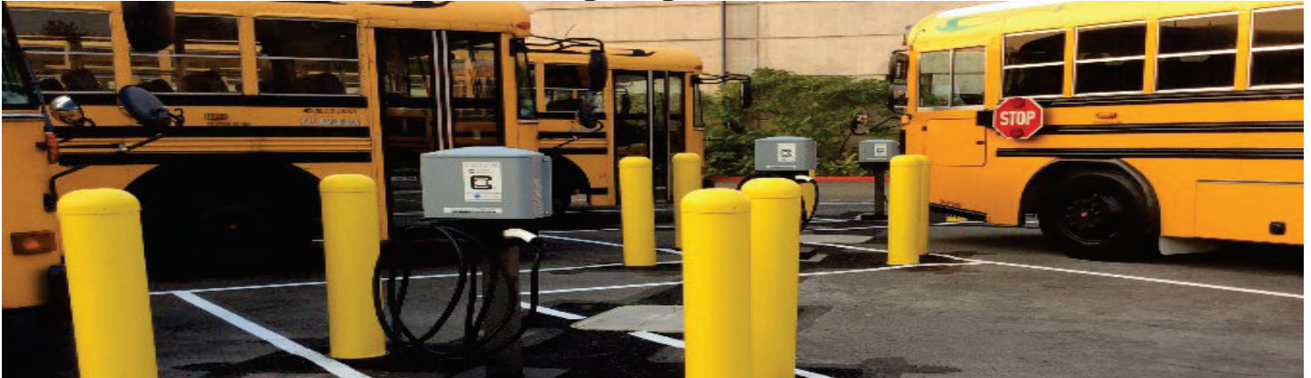
Public school bus fleet charging stations
