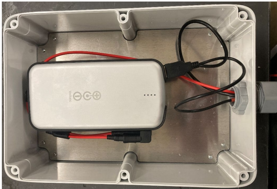
Figure 4. Internal components of the battery enclosure for the Voltaic solar power system (top on left, bottom on right).
