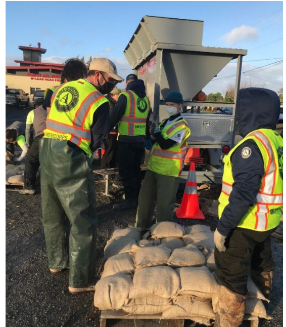
Sandbags filled for flood protection in Skagit County. (Credit: Washington Conservation Corps)
