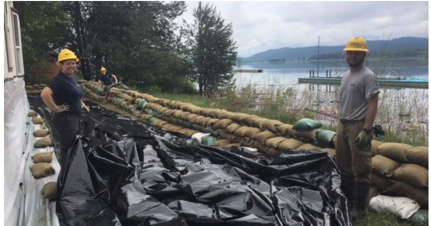
Sandbags being installed to protect a home from flooding. (Credit: Washington Conservation Corps)
