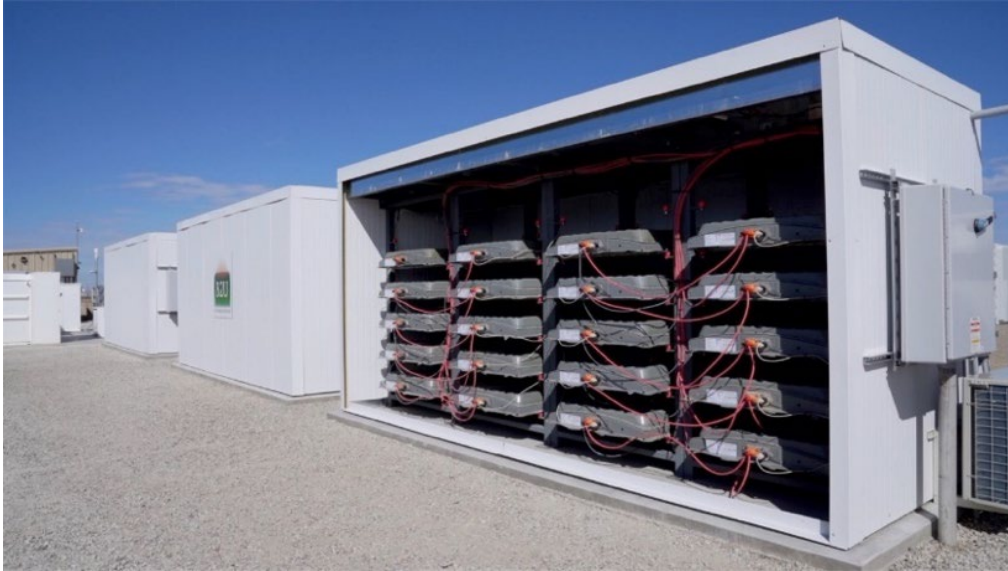
Figure 4. B2U’s UL certified EV Pack Storage (EPS) System enables the use of EV battery packs without reconfiguration in large scale energy storage 17 .
